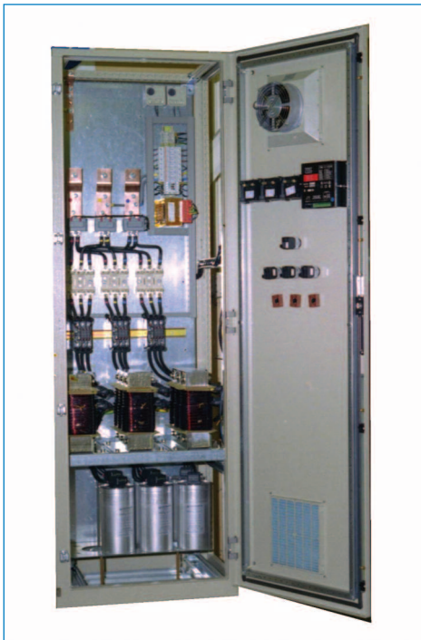
Central automatic power factor correction equipment
