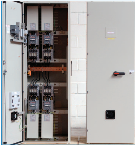
Power factor correction equipment
